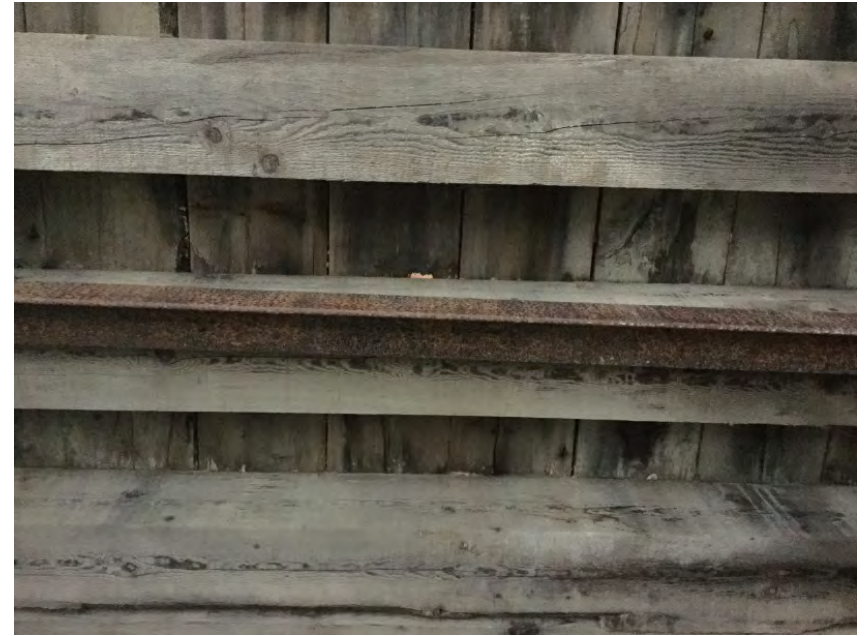
Rot indicators on underside of deck starting to show
